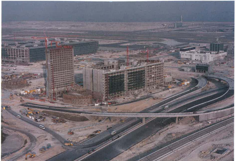
Cathay City – Cathay Pacific's new headquarters – takes shape at the new airport site. 國泰位於新機場的總部。
